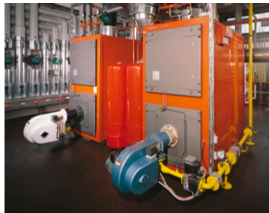
Gas inlet pressure monitoring on high-performance boilers
