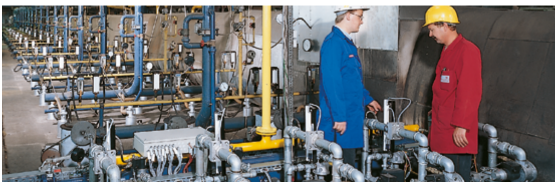
Gas train in a brickworks
